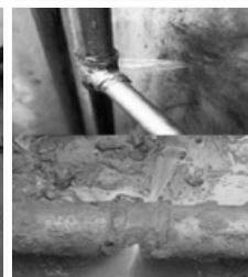
Fire Sprinkler System
