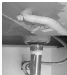
Water Supply Pipe Leakage/ Water Pipe Leakage
